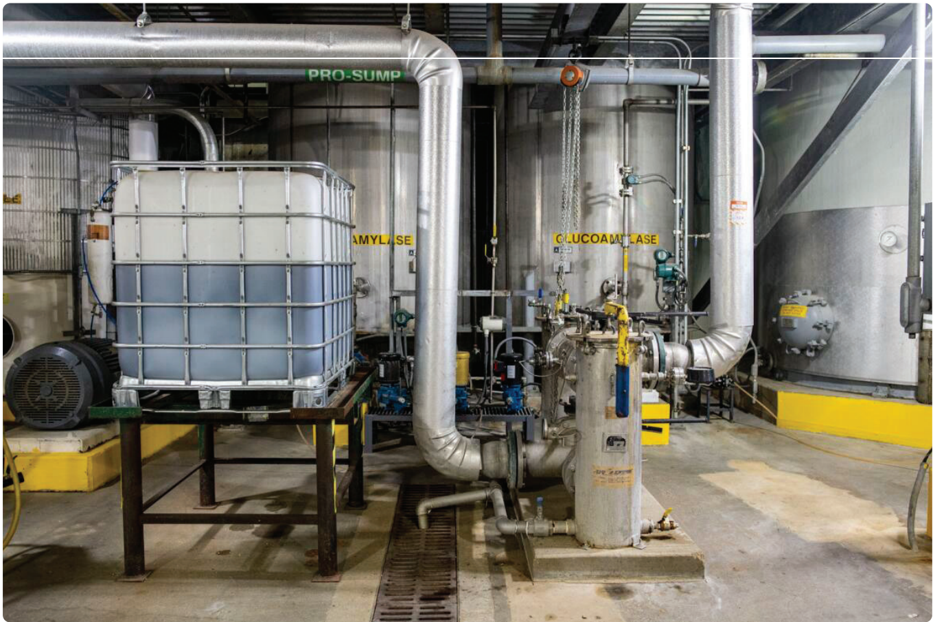
The production line at Atkins Energy's Ethanol and Biodiesel production facility is seen in 2023 in Lena, Ill. (Nick Rohlman/The Gazette)
